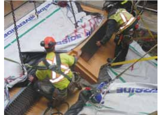
HSK connector at the fully cantilevered atrium stair at UBC Earth Sciences Building. Courtesy of Equilibrium Consulting.
