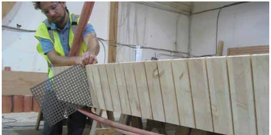
HSK connector being test-fitted for the fully cantilevered atrium stair at UBC Earth Sciences Building. Courtesy of Structurlam Products.
